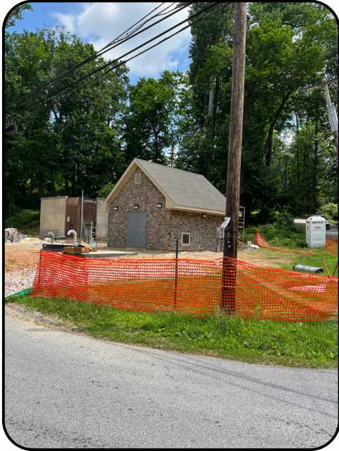
Glenn Avenue Pump Station updates
