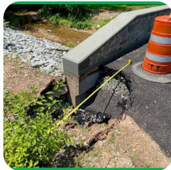
Glenhardie Road Bridge Replacement Project - Sinkhole
